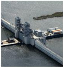
Storm Surge Barriers
