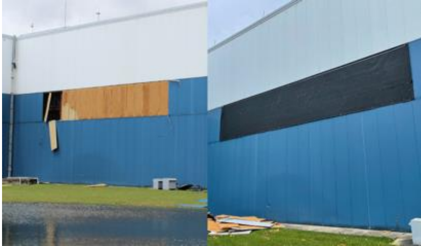
Exterior Siding Damage
