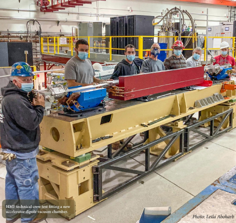
HMF technical crew test fitting a new accelerator dipole vacuum chamber. Photo: Leila Abubahr
